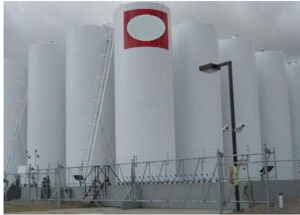
Welded Steel Tank
