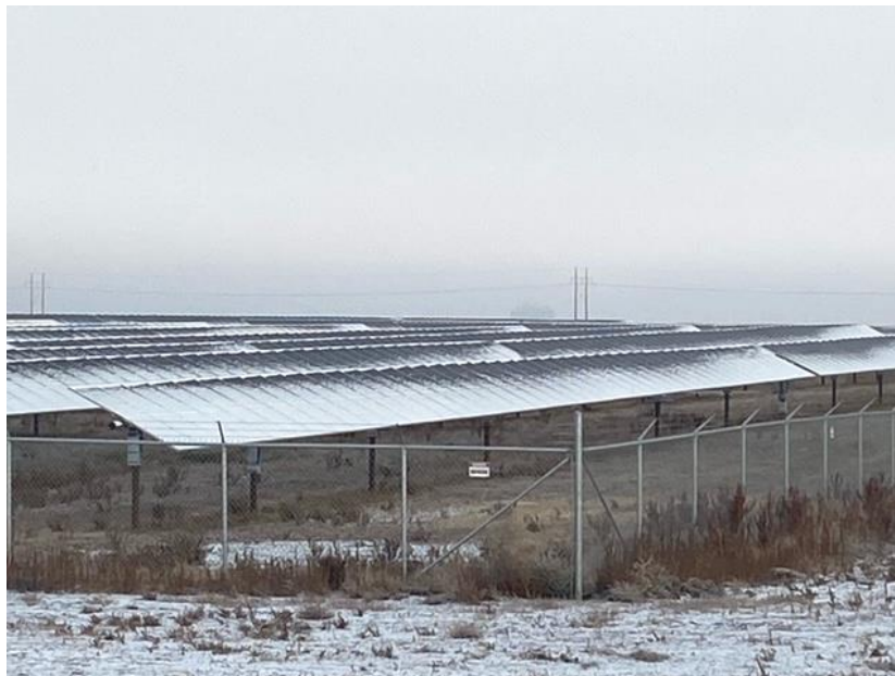
Fixed Tilt Solar Farm (10 MW ac )
